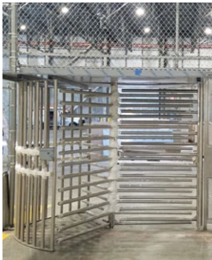
Access Control Systems JFKIA
