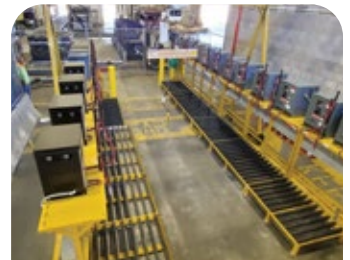
Battery Charging Station JFKIA
