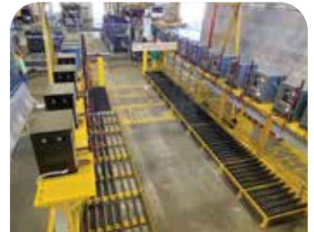
Battery Charging Station JFKIA
