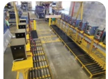
Battery Charging Station JFKIA
