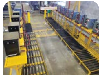
Battery Charging Station JFK Airport
