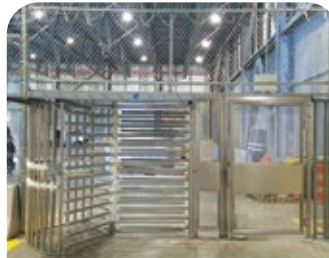
Access Control Systems JFK Airport
