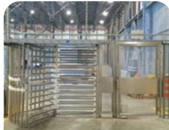
Access Control Systems JFK Airport
