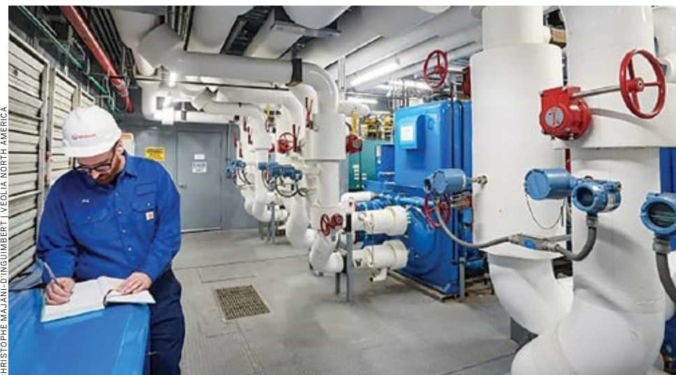
The TWA Hotel at JFK Airport has its own power source. Veolia operator inside TWA Hotel microgrid plant.
