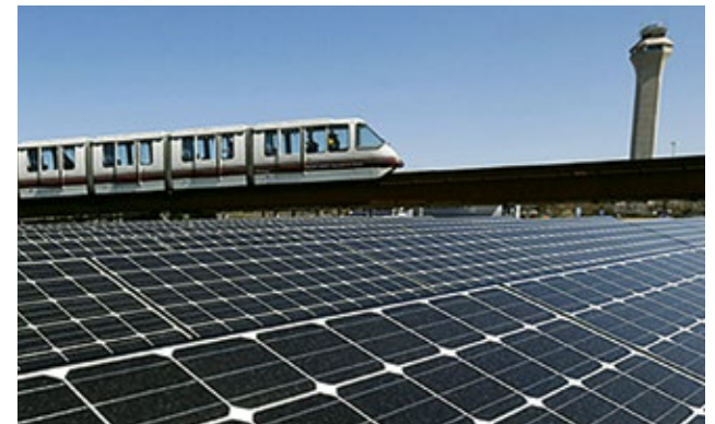
Solar photovoltaic installation at Newark Liberty International Airport.
